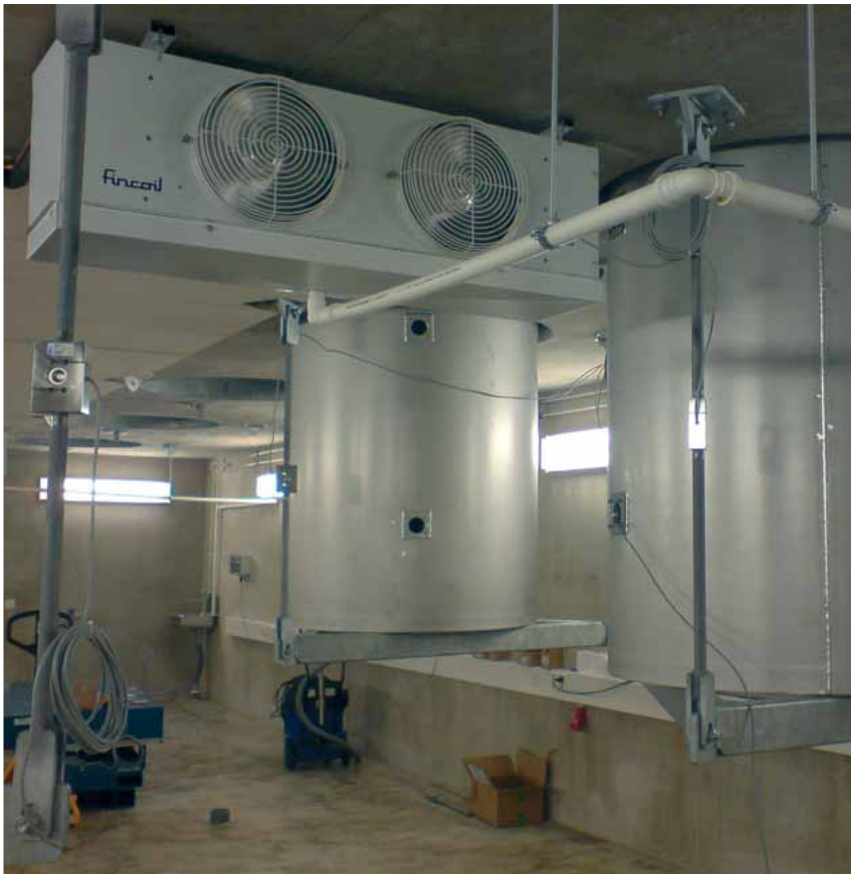
Plant equipment to help control urban flooding and pollution
